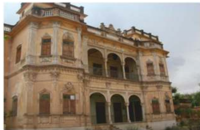
KoolwalKothi :Before Restoration
