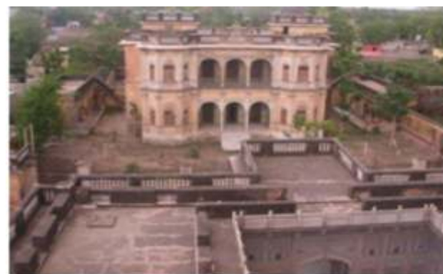
KoolwalKothi :Before Restoration
